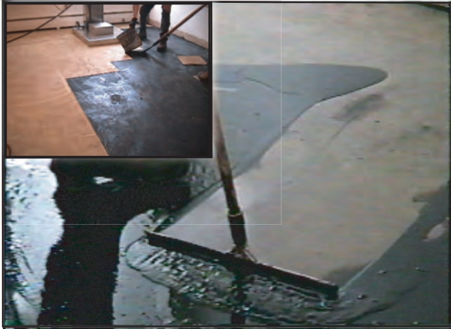
Remove asbestos mastic!
